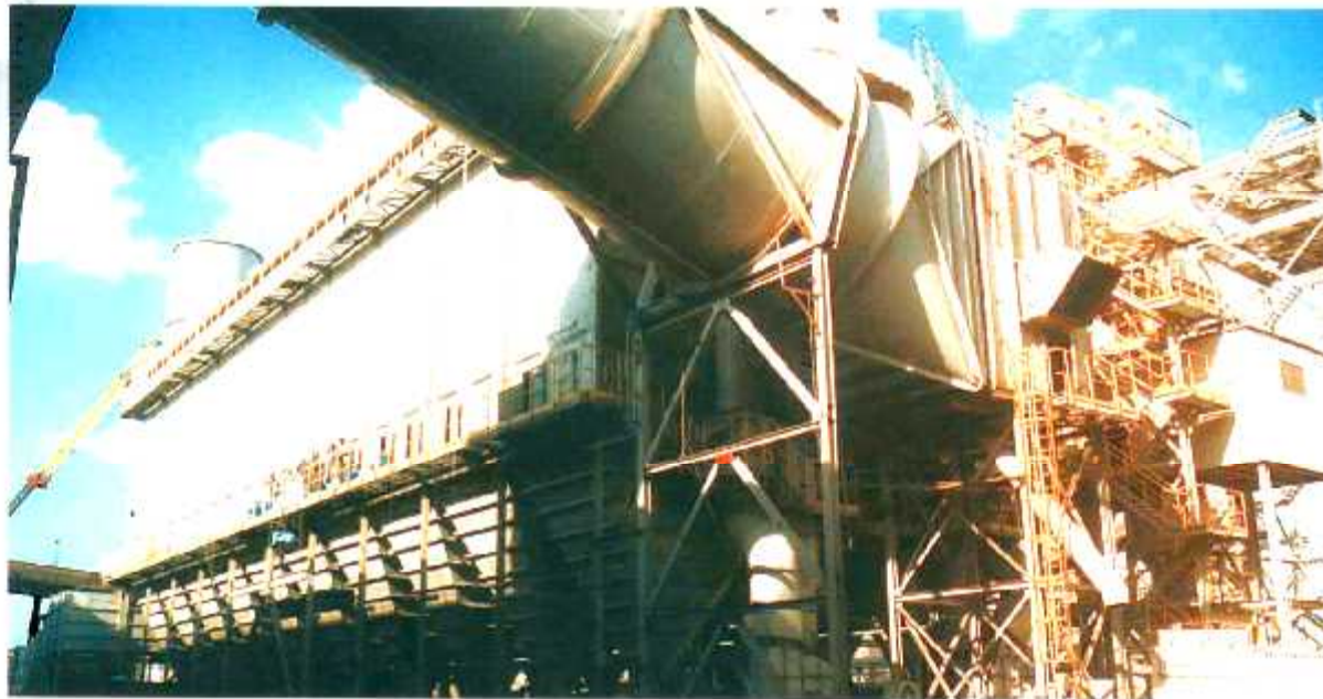
De-dusting in a steel mill Alexandria/Egypt
